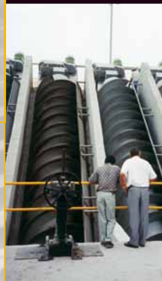
38° foot mounted inclined for Archimedian screw pump - environmental application. NC, USA.
